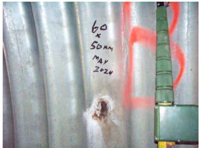
Corrosion on Side wall
