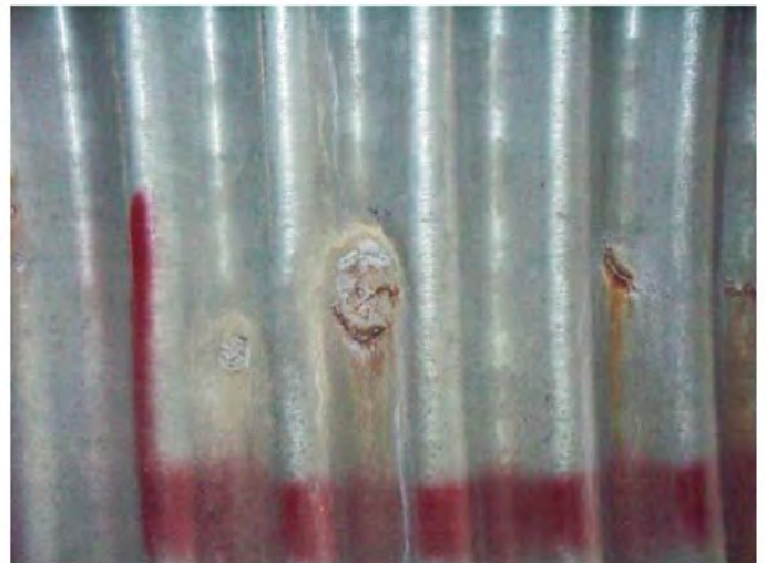
Cracked ring #6 145mm between cracks
